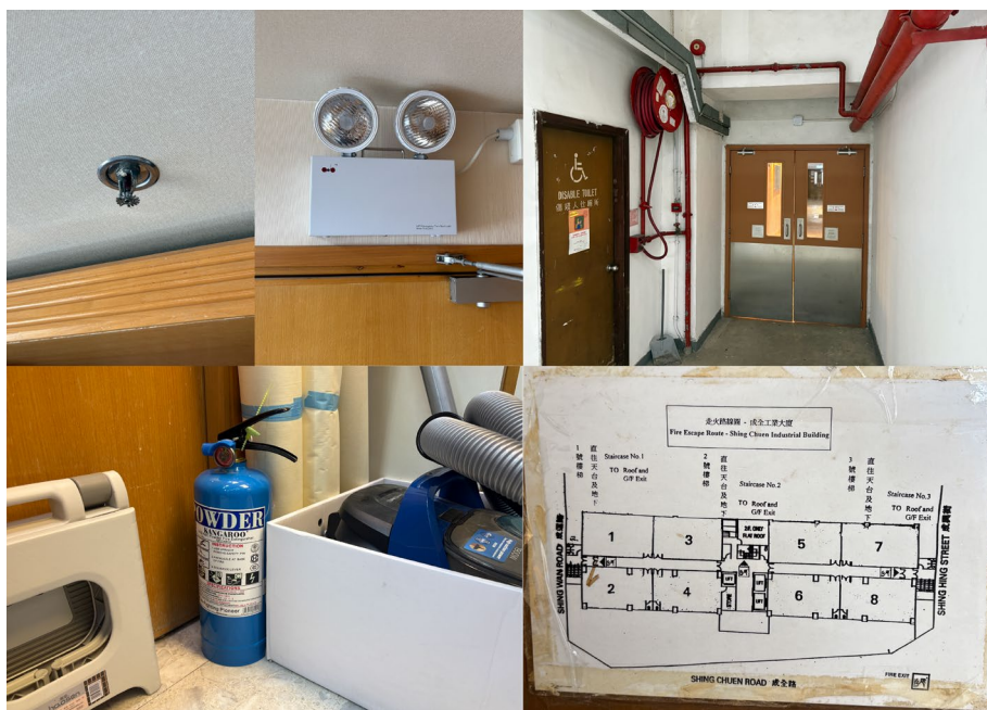
Photo 4.1 Fire Safety Provisions at the Premises and within Shing Chuen Industrial Building
